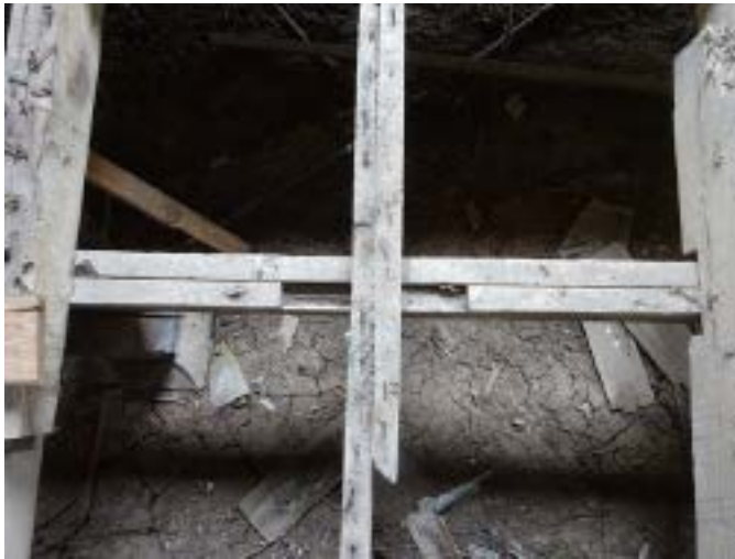
Figure 6. Floor Framing with Unused Mortise and Gable End Cut (Phase 1)
