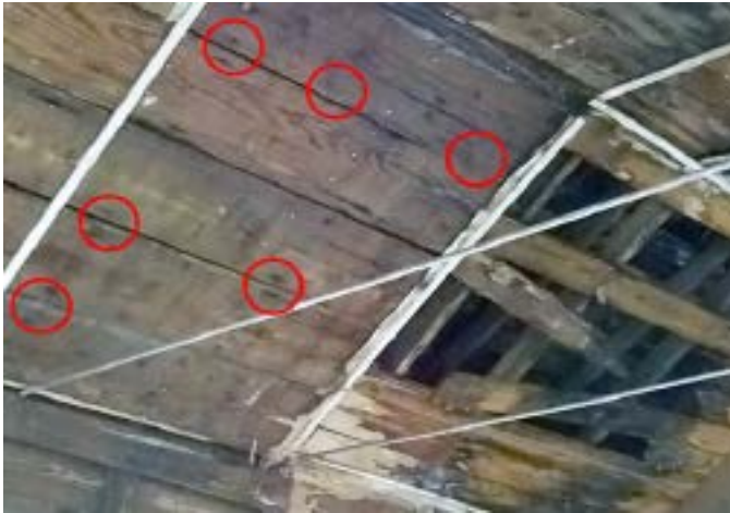
Figure 4. Joint between Phase 1 Meeting Hall and Phase 3 Rostrum Roofs Showing Stains from previous use as the "First" Single-wall Church Source: Image by Michael O'Brien.
