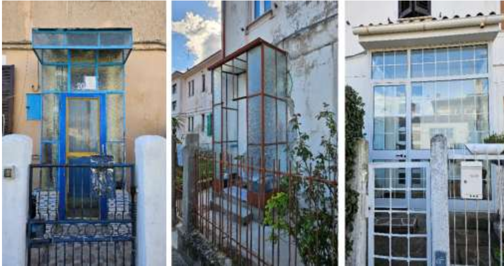
Figure 9. Existing Additions Providing Entrance Protection across Different Building Typologies in Panzano District: The Adopted Protective Systems Vary in both Type and Style
