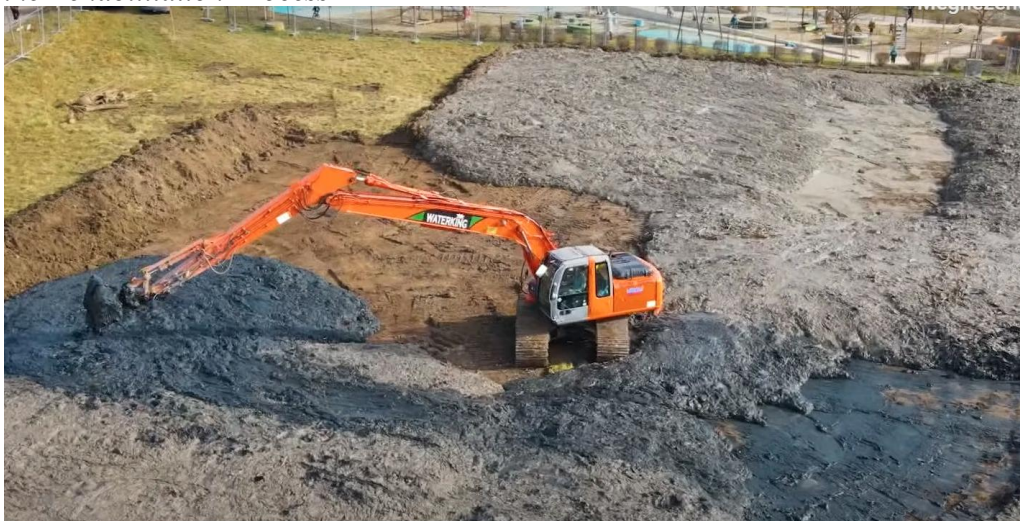
Figure 16. Ongoing Excavation and Drying of Sediment from the Lakes as Part of the Rehabilitation Process
