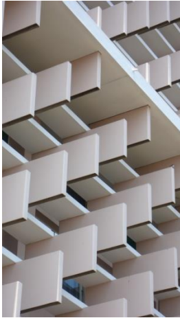
Figure 3. Maristas School, Beira, Mozambique (1959)- Francisco José de Castro. Detail Brise-soleil Source: Ana Magalhães, 2008.
