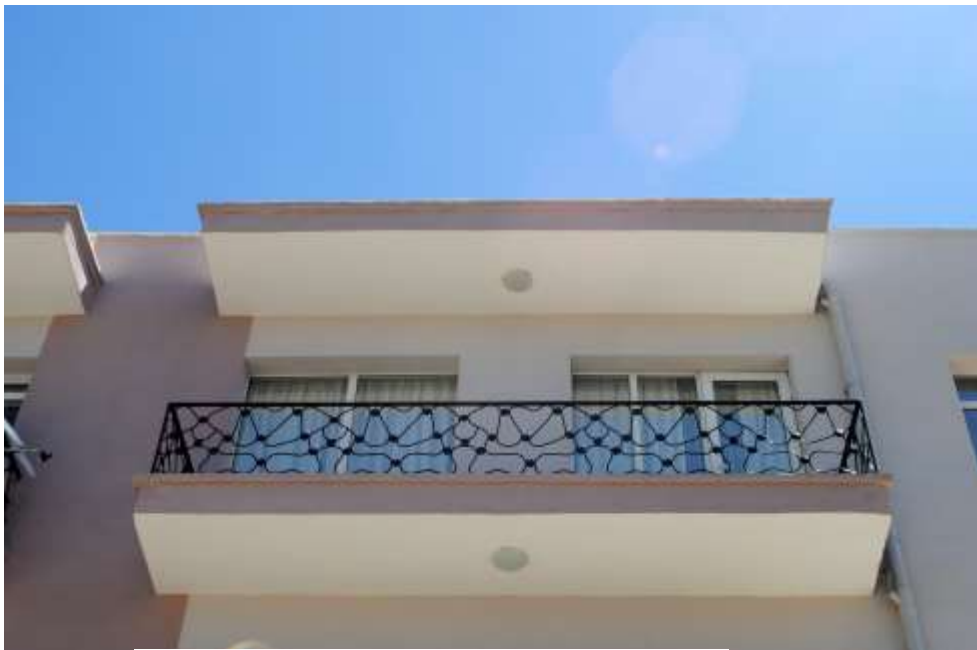
Figure 5. Ankara Balcony Railings, District 3 (Maltepe) Source: The author's archive.
