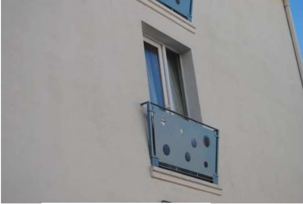
Figure 6. Ankara Balcony Railings, District 4 (Esat)
