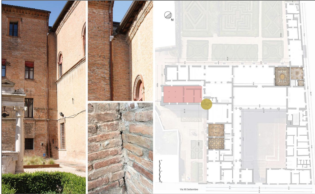
Figure 9. The “Masonry Bandage” (Identified with a Yellow Circle on the Plan) between the Pre-Existing Construction (in Red on the Plan) and the New Construction of Palazzo Costabili to the East
