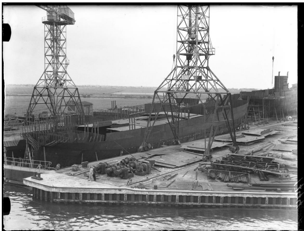
Figure 3. Ships under Construction at the NDSM Shipyard, May 16, 1947. Photo Ben van Meerendonk / AHF, IISH Collection, Amsterdam.
