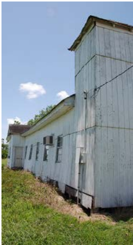
Figure 18. South Wall of South Point Baptist Showing Distortion Source: Michael O'Brien Image.
