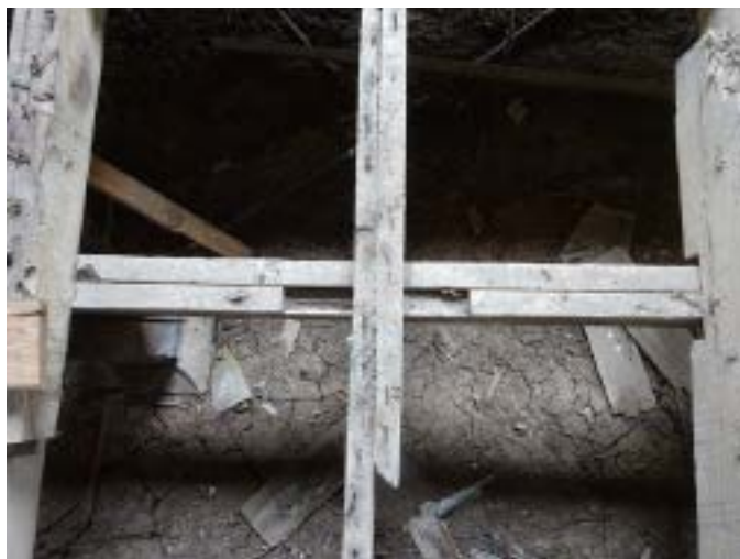
Figure 6. Floor Framing with Unused Mortise and Gable End Cut (Phase 1)
