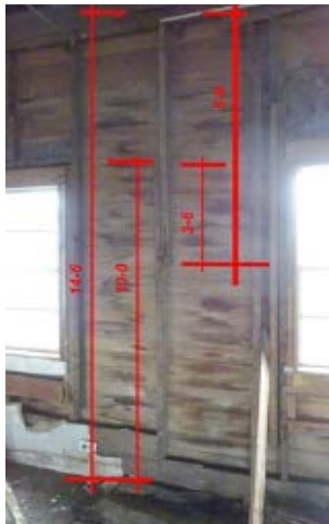
Figure 10. Phase 1 Walls, 8 and 10 Foot Stud "Sistered" to Make a 14'-6 Stud Height Source: Michael O'Brien Image.
