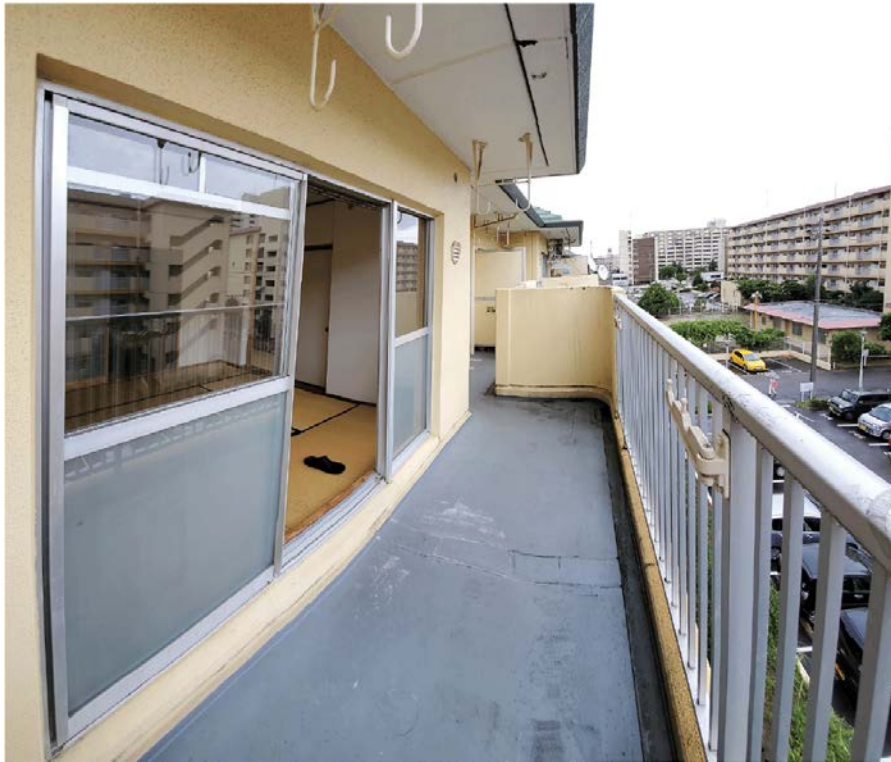
Figure 28. Example of a Balcony in Nagoya Municipal Housing Units which Also Plays the Role of Evacuation Route in Case of Disaster Source: authors.
