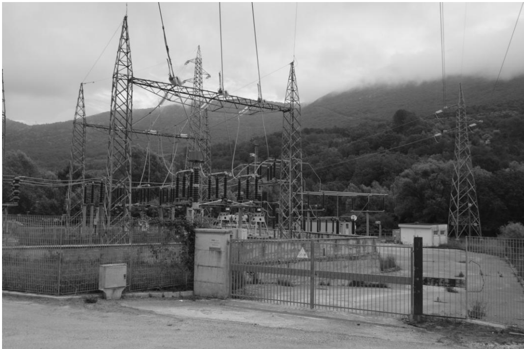
Figure 6. Example of an Outdoor Transformer Station at the Canistro Hydropower Plant, Italy Source: Giulia Azzini 2024.
