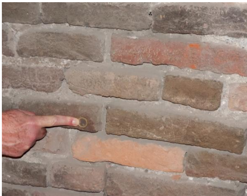
Figure 8. Enlargement of the Window, Vertical Crack Above the Window and Worn Mortar Joints
