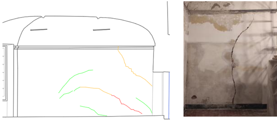
Figure 5. Crack Western Wall in Room B3
