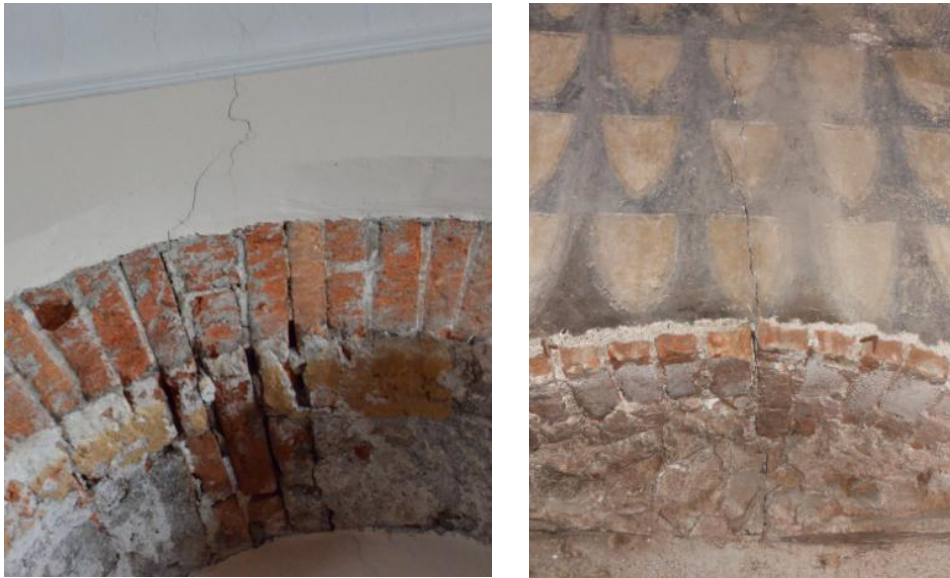
Figure 7. Vertical Cracks on the Opposite Side of the Wall Above the Niches in Rooms C1 (left) and C2 (right)
