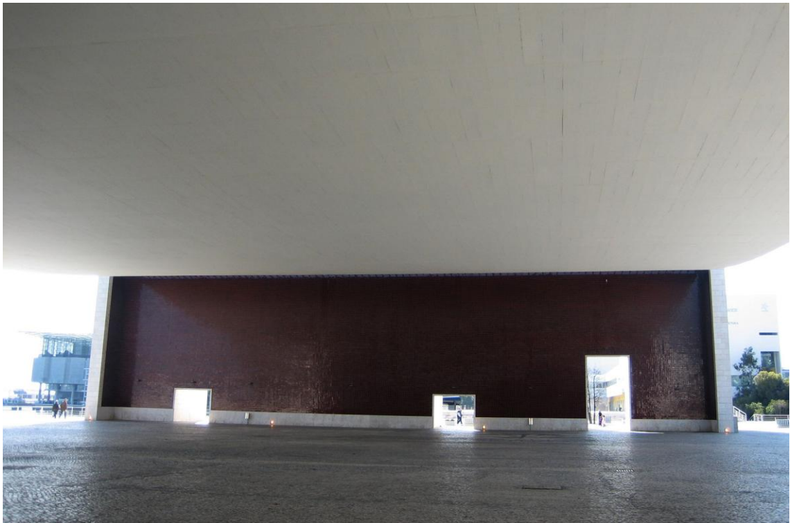
Figure 7. Portuguese Pavilion, underside of the Roof Structure. The Texture of the Maritime Pine ( Pinus pinaster ) Formwork combined with raking Light Produces a “Luminous Vibration” Phenomenon
