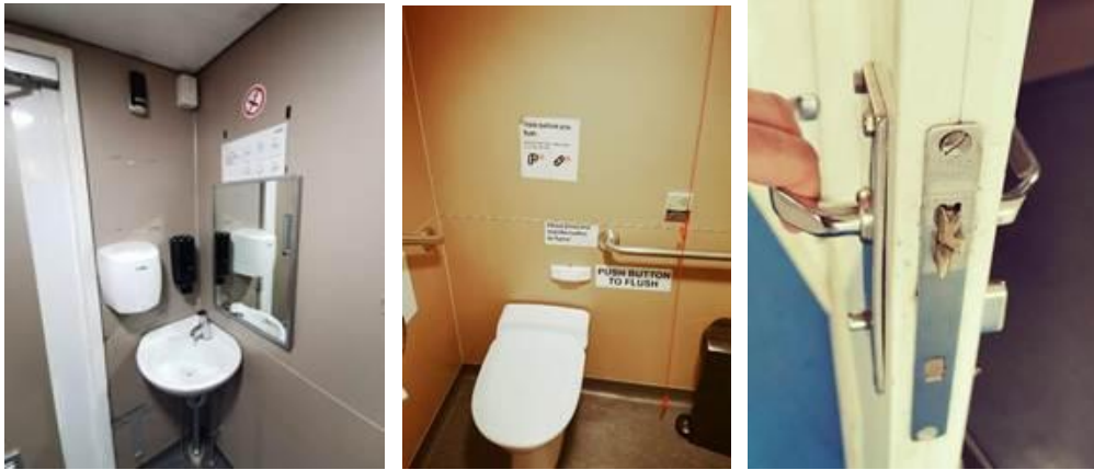
Figure 18. a, b, c. Accessible Restroom Details: Spatial Configuration, Signage, and Door/Lock Elements Affecting Practical Use
