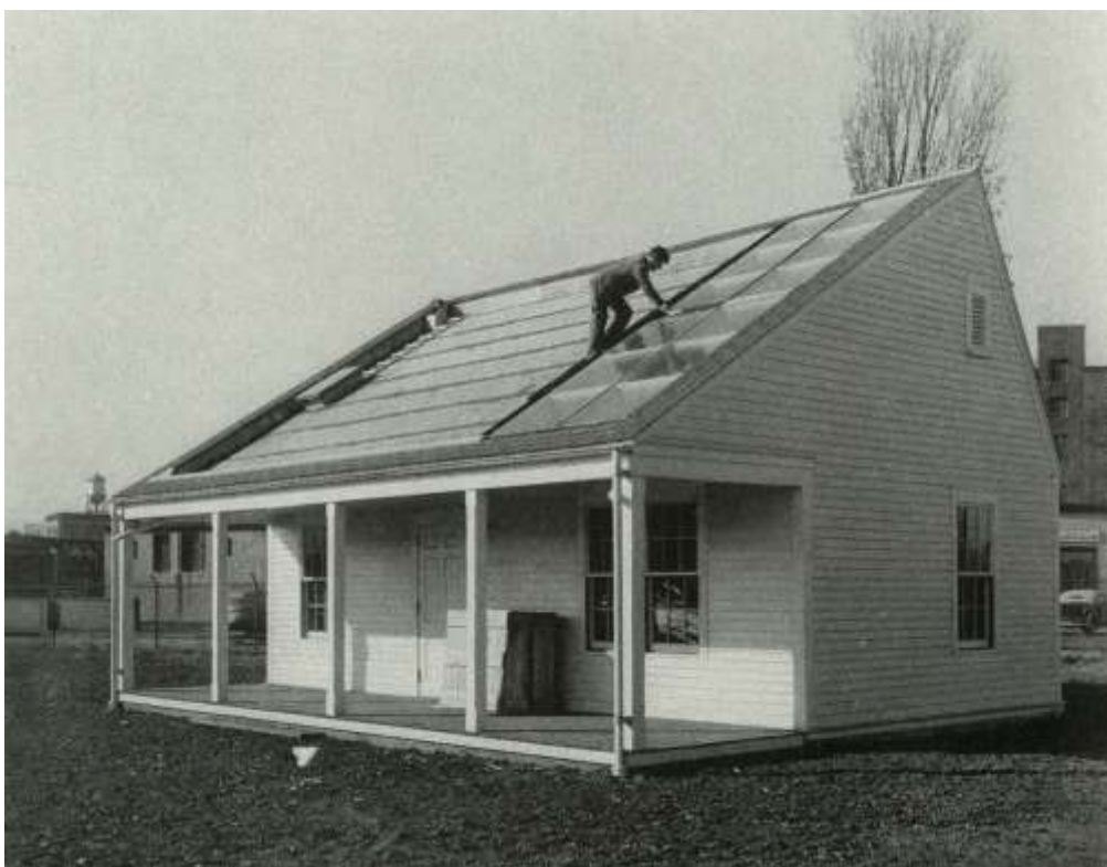
Figure 2. MIT Solar House I, Cambridge, Massachusetts, 1939. Installation of ‘Solar Collectors’ on the Roof of the First ‘Solar House’ Prototype, developed by the Research Group Led by Hoyt Clarke Hottel on the Campus of the Massachusetts Institute of Technology (MIT)
