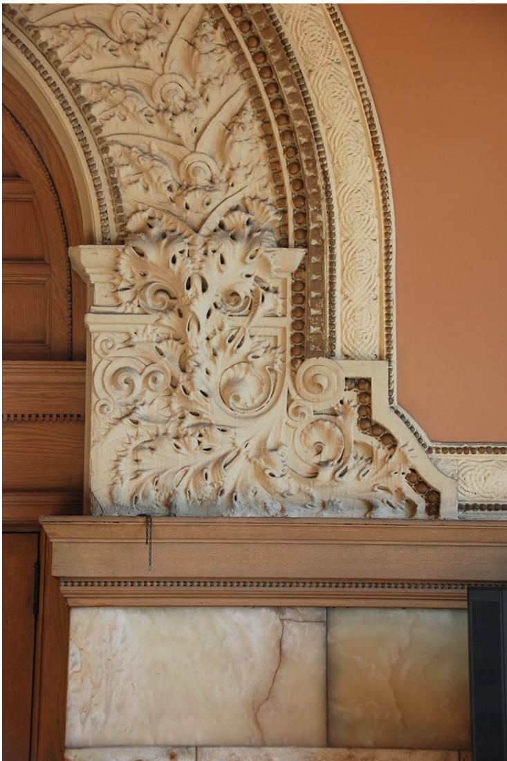
Figure 14. Spring Line Animism-Efflorescence, North Wall Michigan Ave. Lobby Source: Author Photo.
