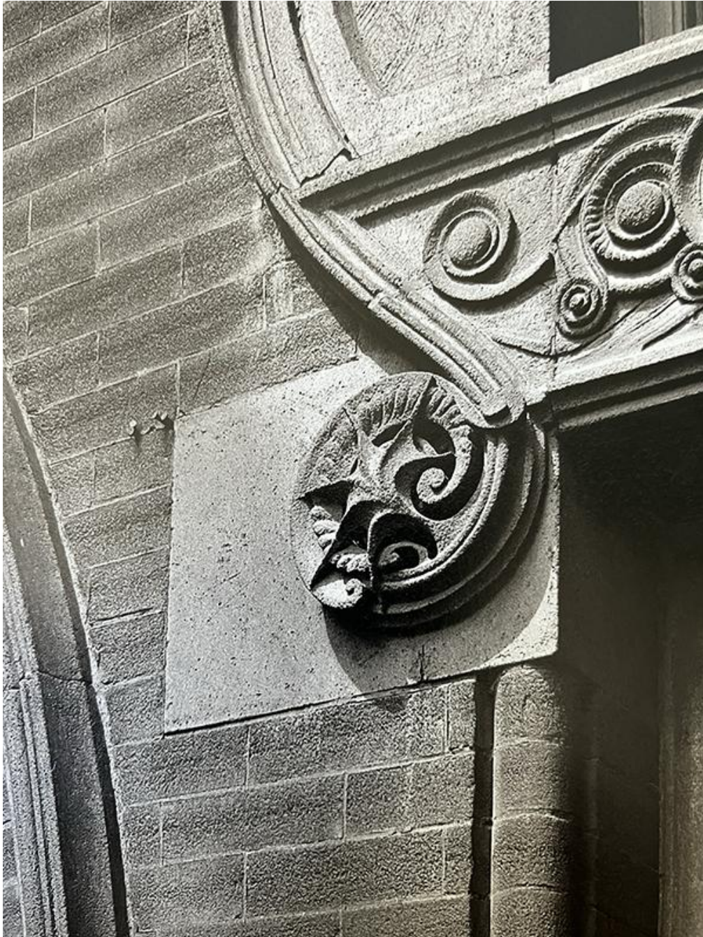
Figure 5. Reuben Rubel House Entry Arch - Extrados Animistic Efflorescence Source: By permission of John Vinci.
