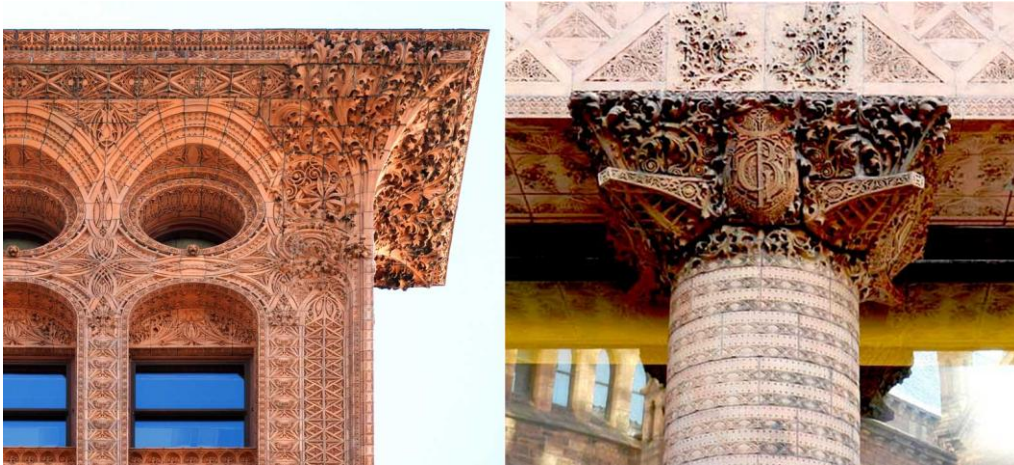
Figure 22. Cornice and Column Capital Efflorescence
