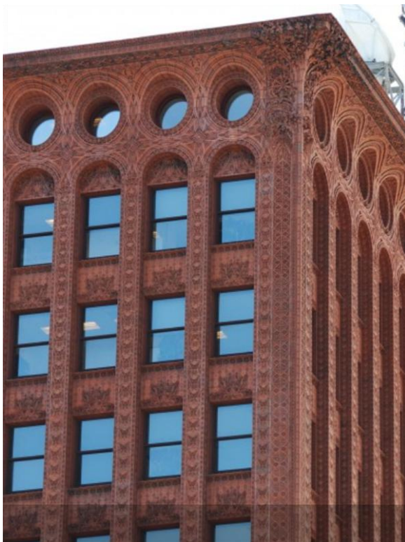
Figure 21. Guaranty Building Cornice - Animistic Efflorescence
