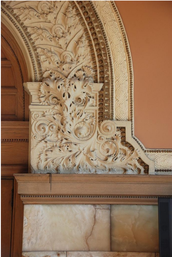
1 2 Figure 14. Spring line efflorescence North wall Michigan Ave. Lobby 3 Photo by author
