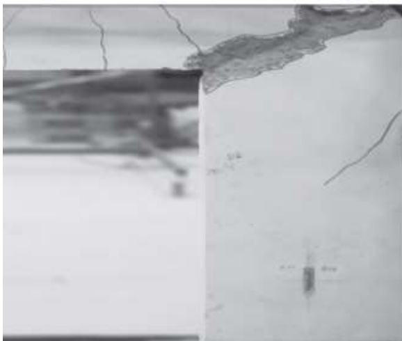
Figure 12. Cracks in Experimental Specimen for I-L
