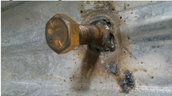
Figure 2. Damages in CFS Steel Plates caused by Welding Process
