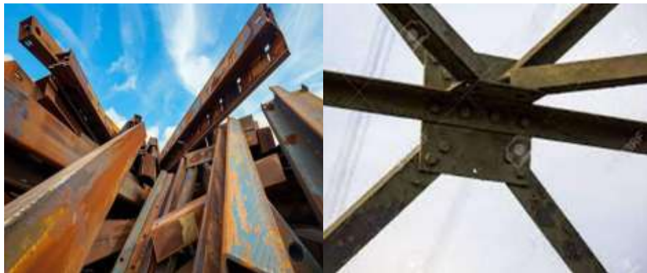
Figure 3. Images from the Experimental Test Set: Steel Construction with Corrosion
